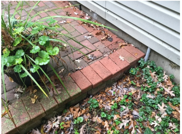
loose bricks at patio were noted
